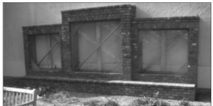
The St. James Columbarium framing. By press time, the flagstone, copper flashing and niches should be installed.
